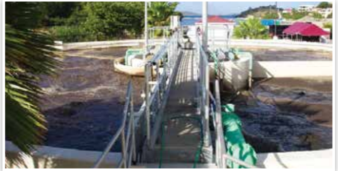
Circular Field Erected Plant For Flows up to 1,000,000 GPD
