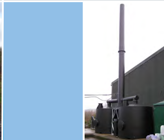
▲ 2 No. carbon filter and emission stack for a styrene abatement plant
